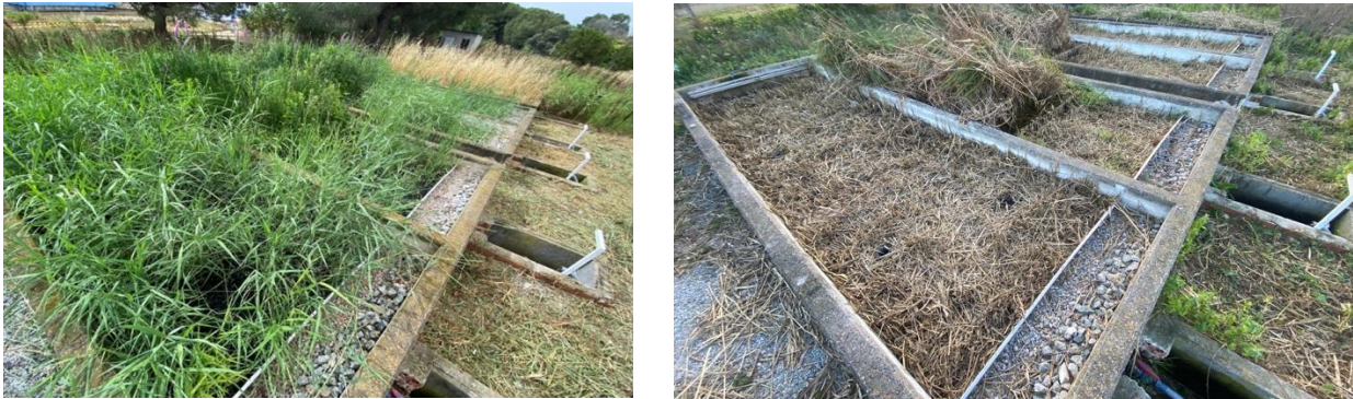
Figure 17. Photos of the pilot plant showing the four different treatment units during the warm and cold season.
